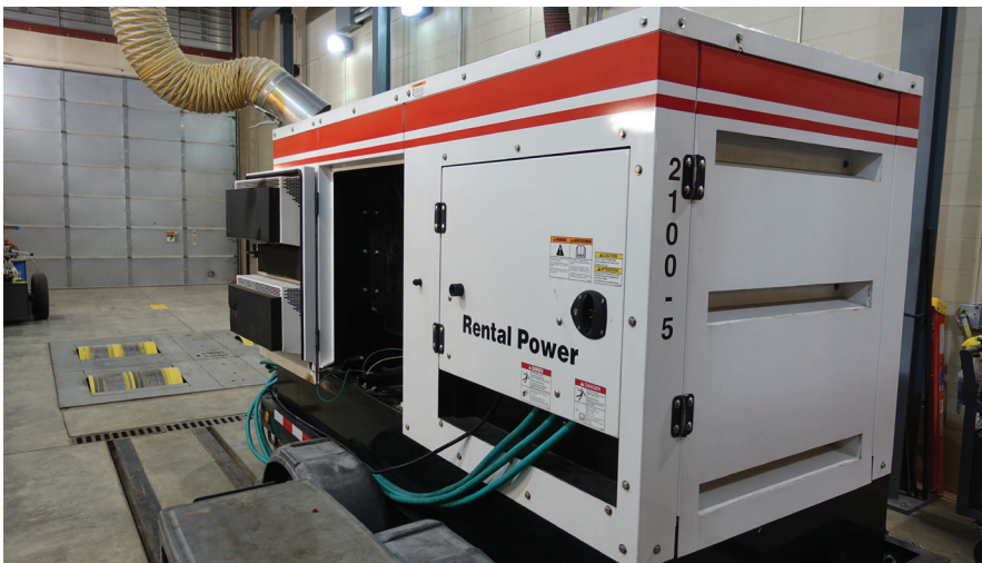
Generator set in the Horton Chassis Dynamometer Room at Horton
